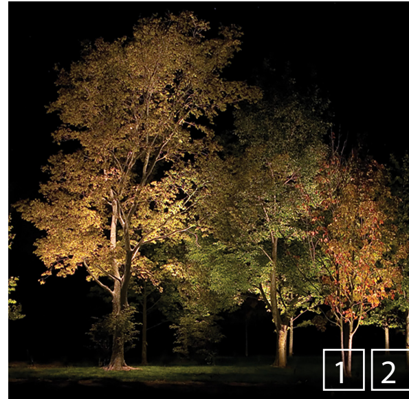
TREE MOUNTED DOWNLIGHTS ADJUSTABLE ACCENTLIGHTS INTEGRATED INTO TREES A WITH WIDE BEAM TO PROVIDE INTERNAL GLOW TO TREE CANOPY
